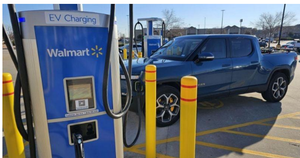
Figure 2.2 Walmart EV Charging Station, Source [48].
