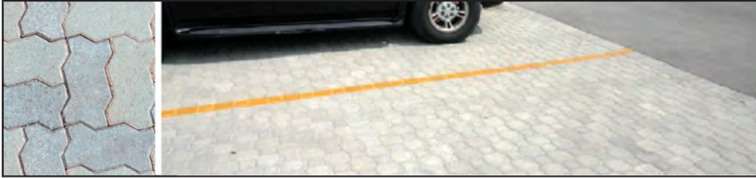
Figure 2-60. High albedo, interlocking block pavers. Photo courtesy of LCRA Service Center, Austin, Texas.
