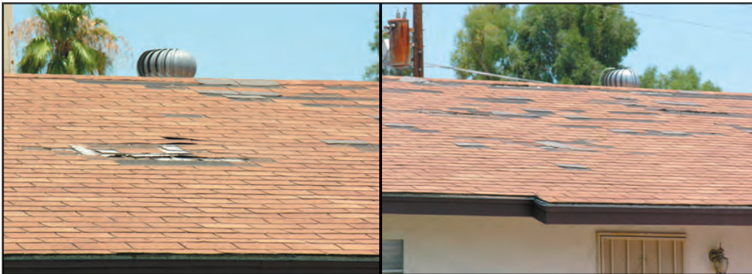
Figure 2-40. Examples of deteriorating asphalt shingle roofs on residential homes in Phoenix. Photos courtesy of National Center of Excellence, Arizona State University.
