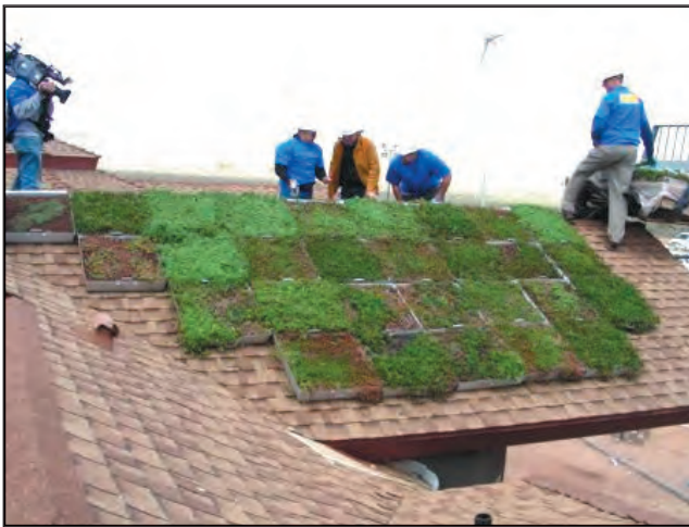
Figure 2-37. Modular, extensive green roof being constructed on a sloped residential home in Pinon, Arizona. Source: www.greenroofs.com.
