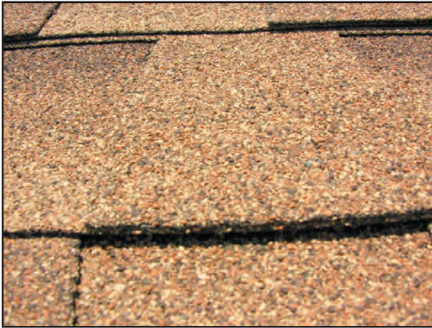
Figure 2-18. Common asphalt shingles up close. Photo courtesy of National Center of Excellence, Arizona State University.
