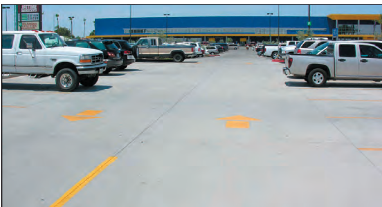
Figure 2-57. Portland cement concrete parking lot in Tempe, Arizona. Photo courtesy of National Center of Excellence, Arizona State University.
