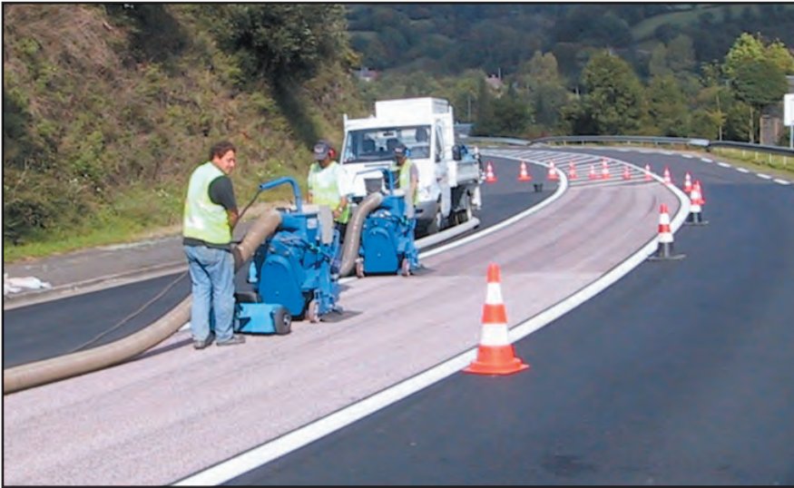
Figure 2-65. New technologies such as shot-blasting are being developed to lighten asphalt pavement immediately after construction. This technique abraded the surface binder. Photo courtesy of the Asphalt Pavement Alliance.
