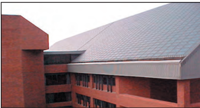
Georgetown University Intercultural Center in Washington DC exemplifies a roof integrated PV system. Photo courtesy of Georgetown University
