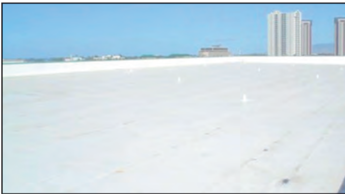
Figure 2-33. Cool-roof, PVC, single-ply membrane applied to a roof. Photo courtesy of Honolulu Roofing Company.
