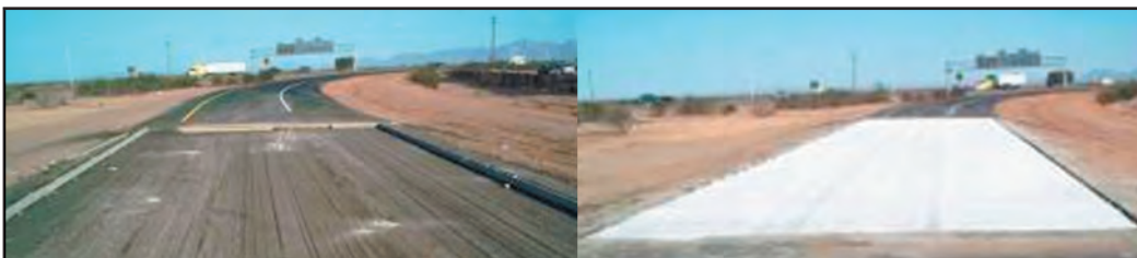
Figure 2-59. A thin white topping project in Phoenix: (a) grinding down the existing asphalt base, and (b) curing the final surface. Photos courtesy of National Center of Excellence, Arizona State University.
